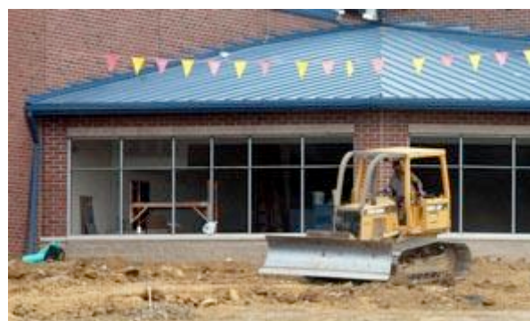
A construction worker moves dirt near the front of Clark's Run Road. The board of education Monarch Construction contractor until construction is acceptable. Bri
